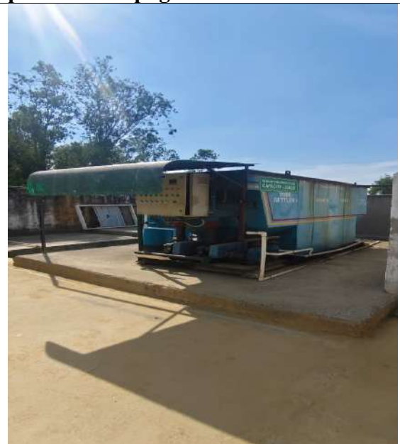
Photograph of STP installed in unit
